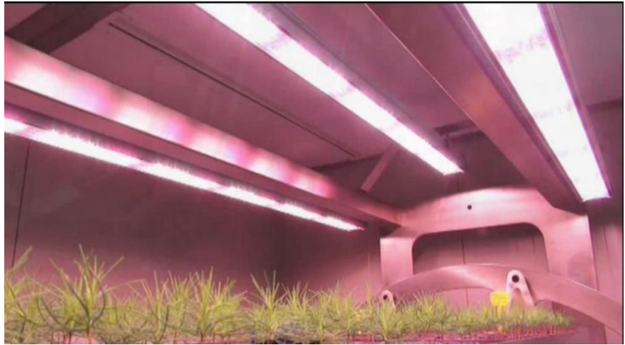
Figure III: three rows of special LED lamps inside the Zephyr growth chamber
