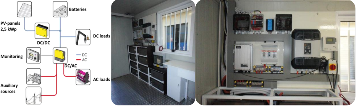
Figure 2: Basic Power system design and final installation
