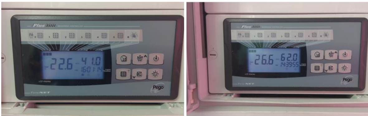
Figure 1 HVAC control unit
