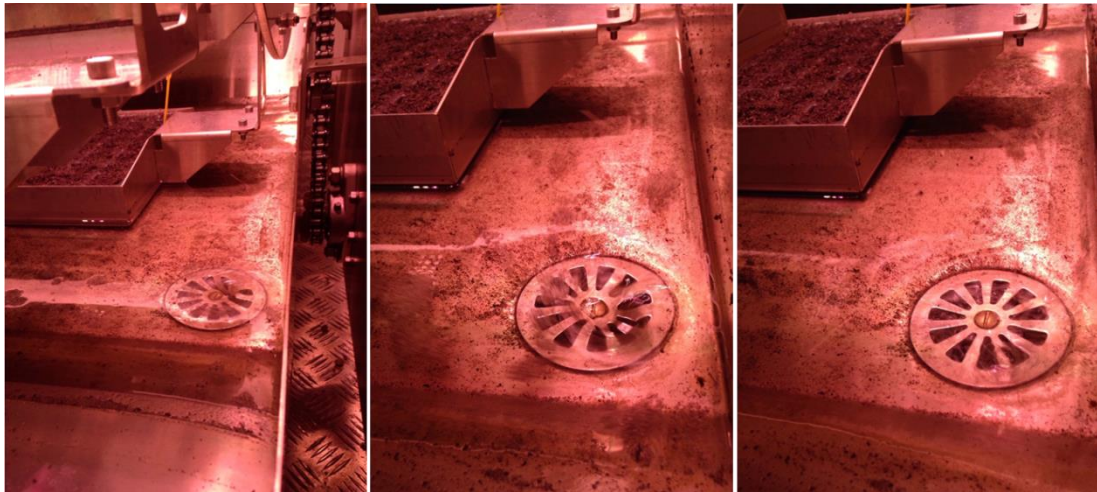
Figure 12 Draining valve opened
